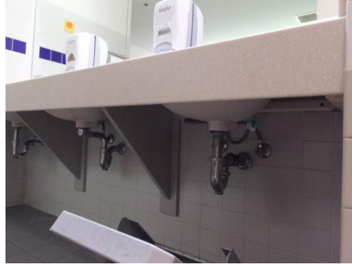
Figure 31 - Typical Hot Water and Drain Pipes without Insulation (Men's Room on Main Level Exhibits Area)
