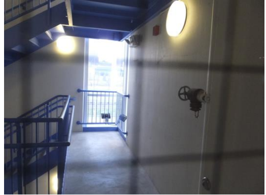
Figure 27 - Sprinkler Stand Pipe Valves are not Cane Detectable in Exit Stairs
