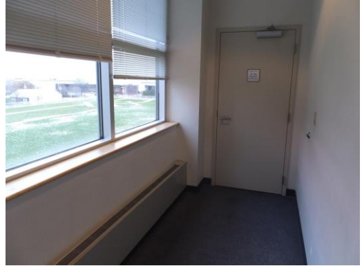
Figure 25 - Limited Maneuvering Space on Pull Side of Exit Door in Polymer Funhouse Area
