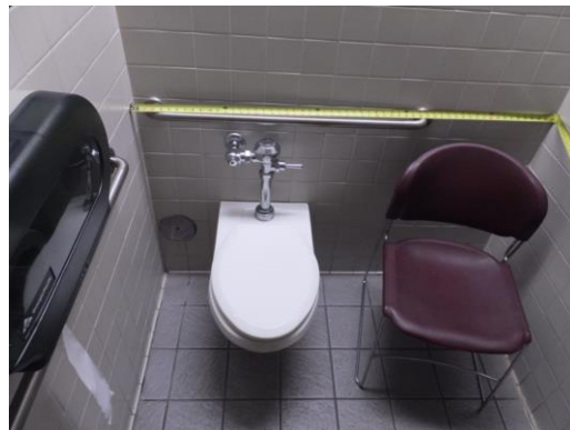
Figure 32 - Accessible Stall too Narrow (57-1/2") in Women's Main Level Exhibit Area
