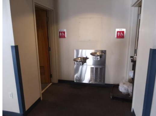
Figure 29 - Drinking Fountains Block Access to Restroom Doors at Upper Level Exhibits Area
