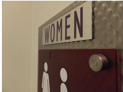
Figure 28 - Typical Restroom Signs Lack Raised Letters as Required by UFAS
